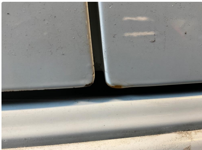
1.1 Rust i fals.
