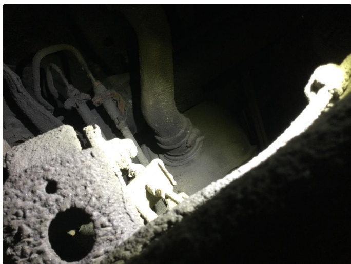
1.2 Noe rust, anbefaler behandling
