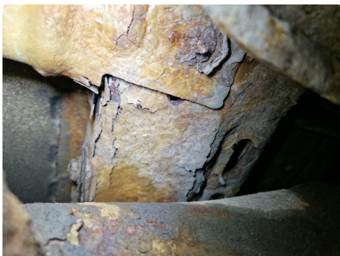
1.1 Rust underside bil.
