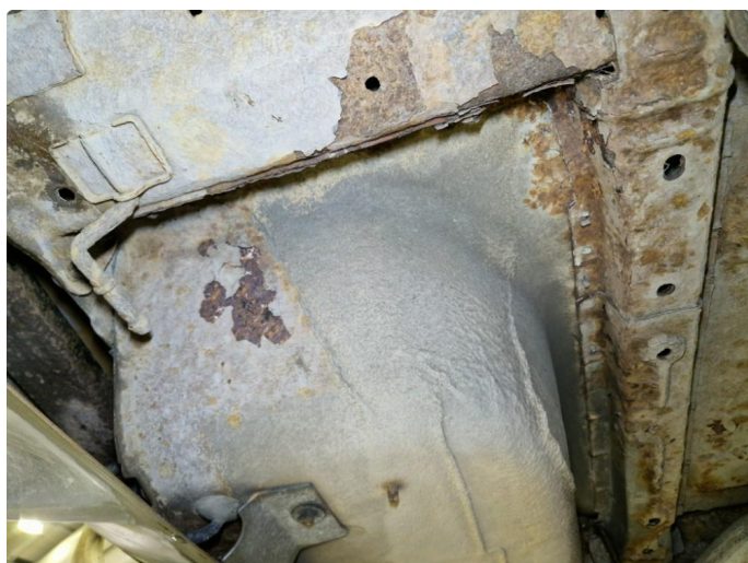
1.1 Rust underside bil.
