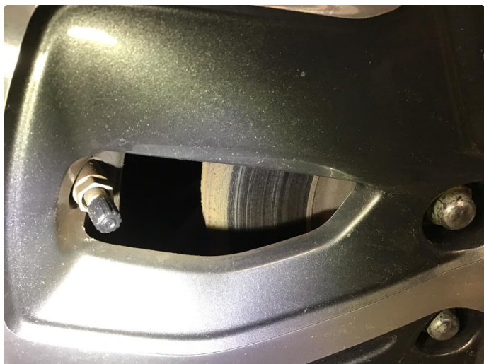
2.1 Mer enn 25% rust
