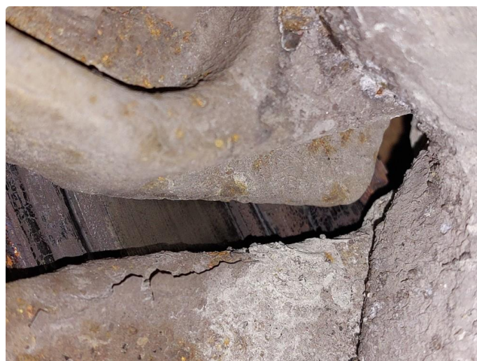
4.3 Mer enn 25% rust
